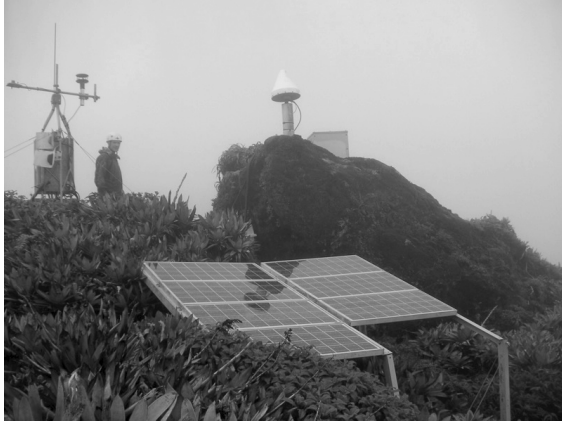
Fig. 5. Example of power and transmission equipment for the permanent station Sanner operating at the summit of La Soufrière in Guadeloupe. The solar panels have a nominal power of 378 W for a power consumption of 20 W. The buffer accumulators have a capacity of 300 A h. No power failure has ever occurred at this station during 8 years of continuous operation.
